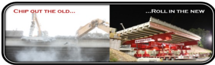
Rehabilitation of Bridge Numbers 01235 and 01236, Interstate 84 over Marion Avenue in Southington DOT Project No. 0131-0194/195
